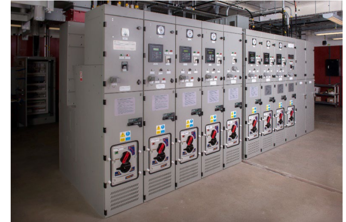
DC Switchgear Line Up
