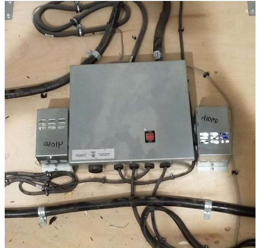
Top of Car Control & LEDs
