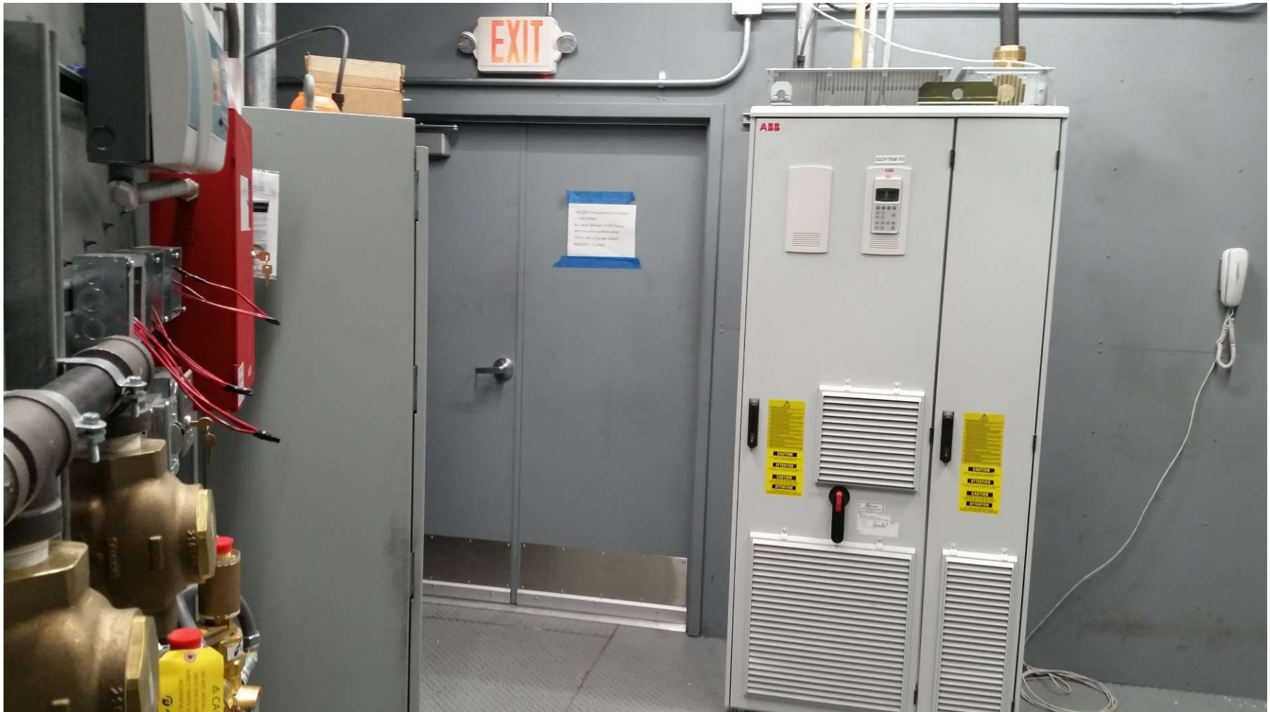
VFD at the St. Louis Arch
