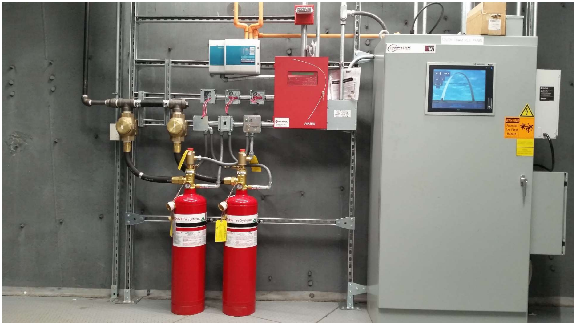
PLC Cabinet and VFD Room Fire Suppression System At the St. Louis Arch
