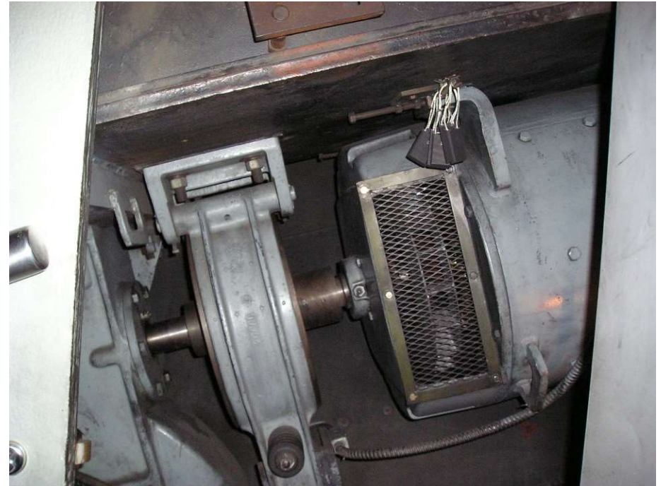
DC Motor and Brake Replaced in 2016
