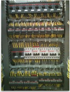
HVAC Control Panels
