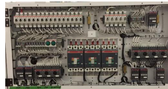
Control & Distribution panel
